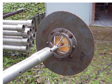
Figure 13: Packed flow meter [Wiacek 2003]
